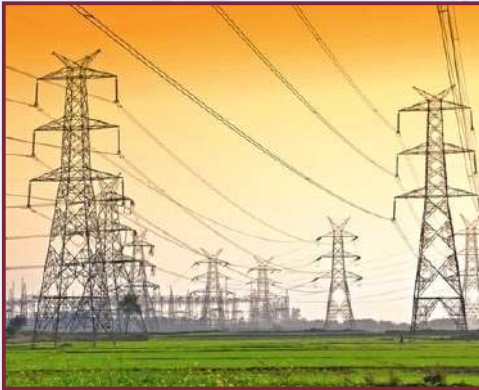
EXTRA HIGH VOLTAGE 132kV to 400kV
