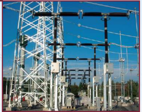
ULTRA HIGH VOLTAGE 400kV to 765kV
