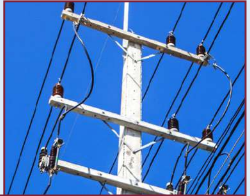
MEDIUM VOLTAGE 11kV to 66kV
